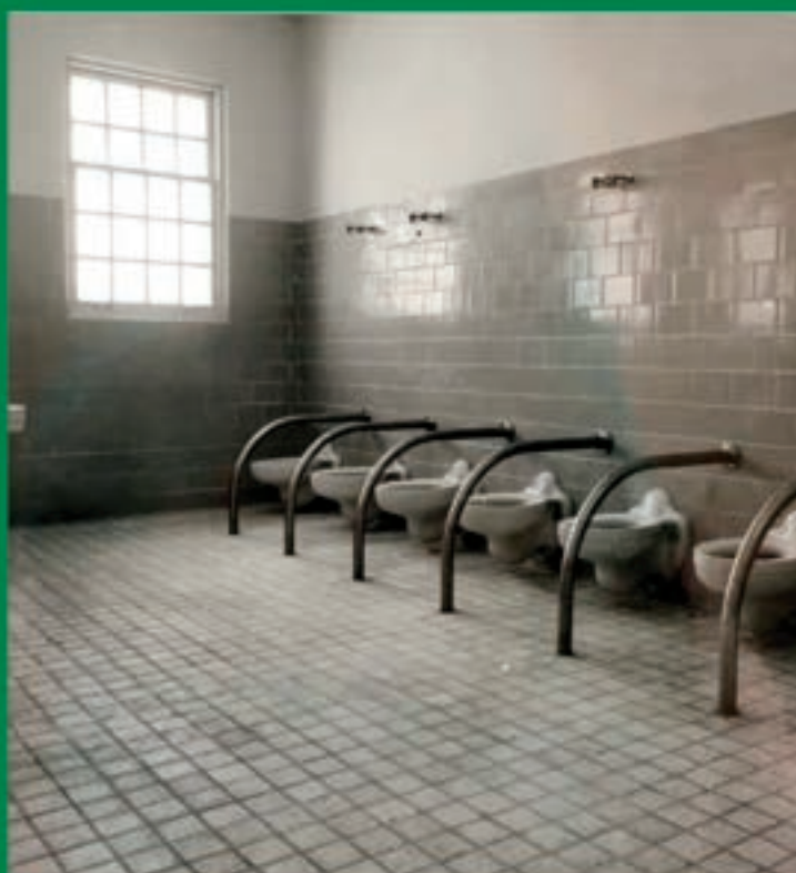
Photo of the Manitoba Development Centre's toilet From Online News Article: "$50M lawsuit alleges intellectually disabled residents were sexually abused, starved at Manitoba institution" by Laura Glowacki for CBC, December 19, 2018
